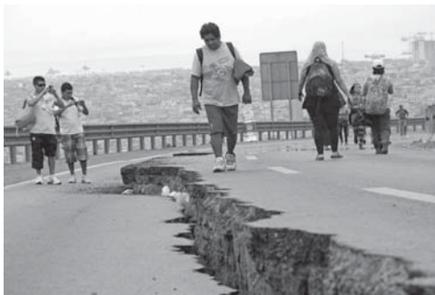
Fig. 4 Ruptured road in Iquique (ABC News)
