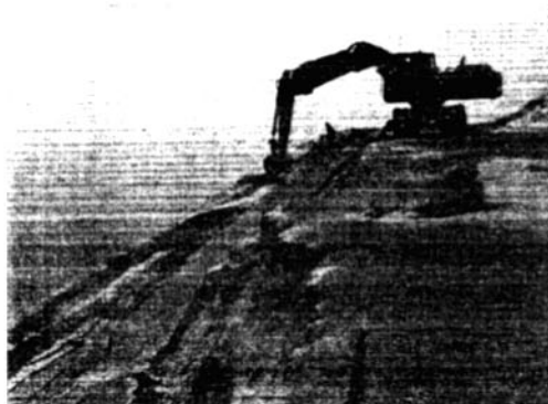
Figure 3 Damaged Pan American Highway near Ocona.
